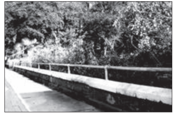
The concrete fence at the 1911 Gwynne Institute at Second and Jackson was constructed soon after the building was finished
